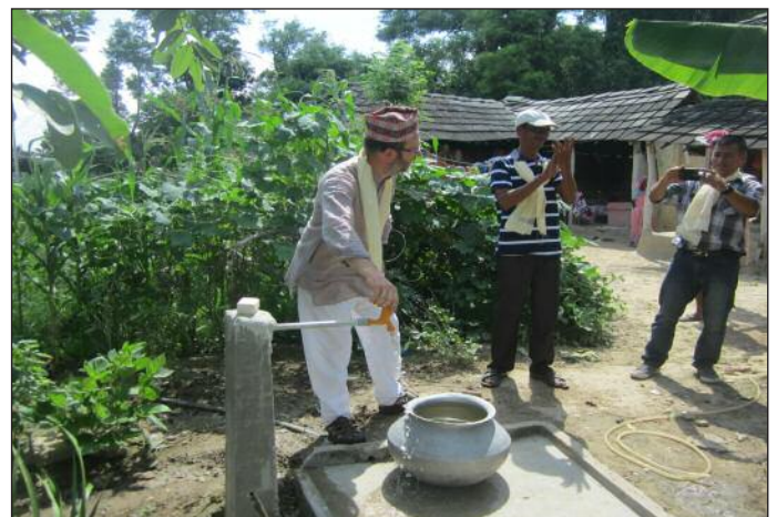
TUI member, Mike Winterburn of Limerick Colleges Branch, sent in an application on behalf of the Nepal Leprosy Trust in 2015 and 2016. Funds went towards water and sanitation work (pictured above) and the construction of a community hall.
